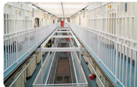
Refurbished prison wing following redecoration and lighting, electrical and flooring upgrades, HMP Liverpool
